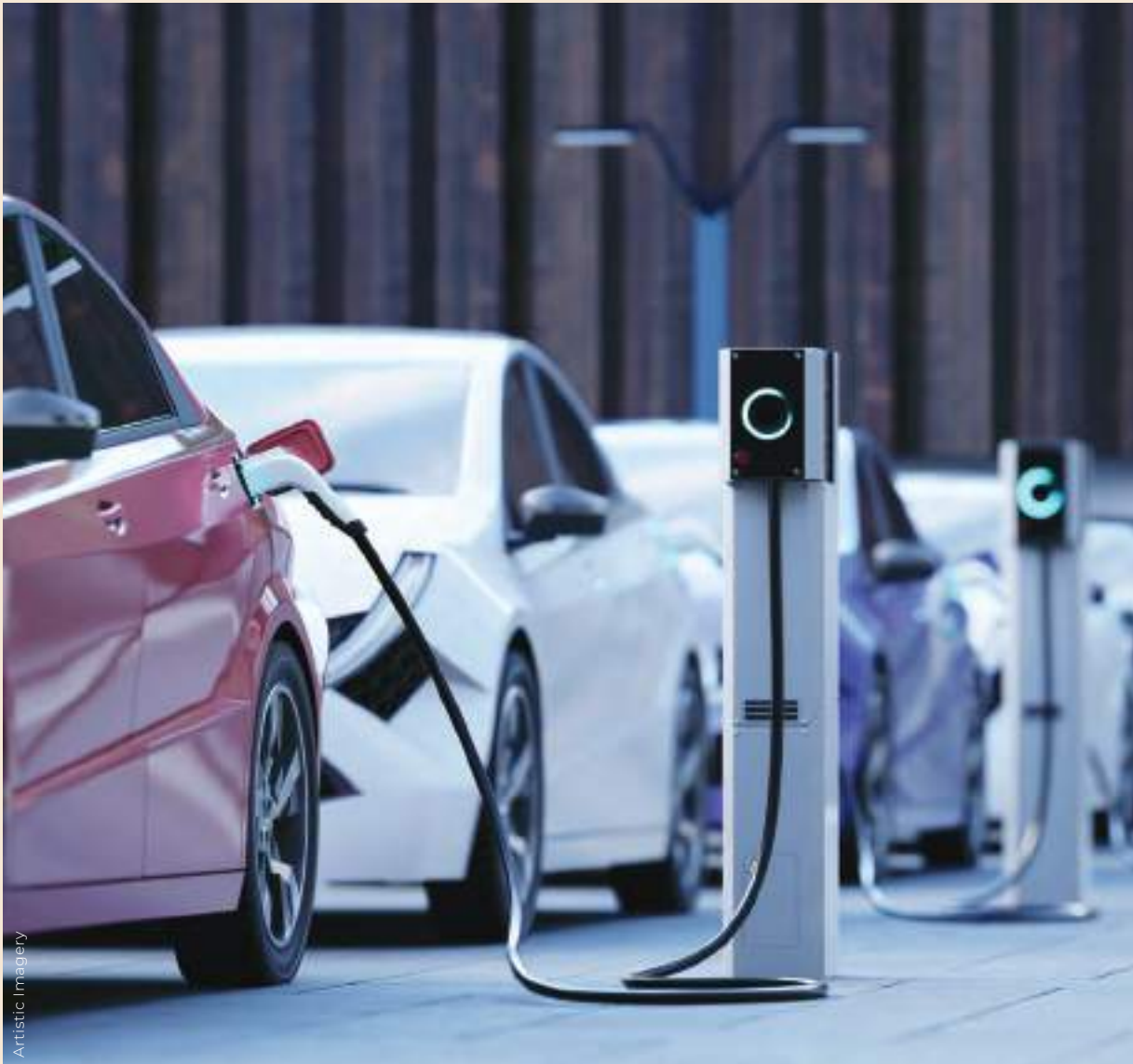
EV Charging Stations
